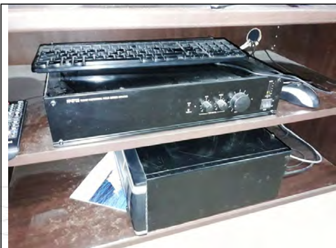
77. sound station 2W EX TPOLYC7800-122
